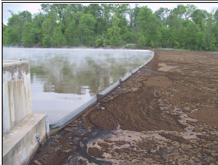
Figure 3: Floating baffle fitted with filtering flow through windows to limit sludge movement in pond
