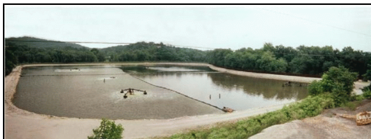
Figure 1: Typical floating baffle installation dividing a waste water pond into four treatment cells. Flow is controlled between each cell through the use of flow through windows.
