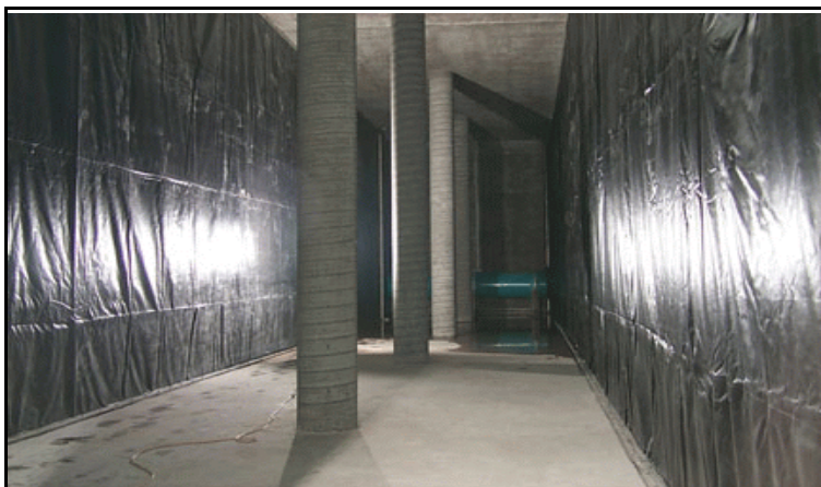
Figure 2: Typical fixed baffle curtain located inside a water treatment facility
